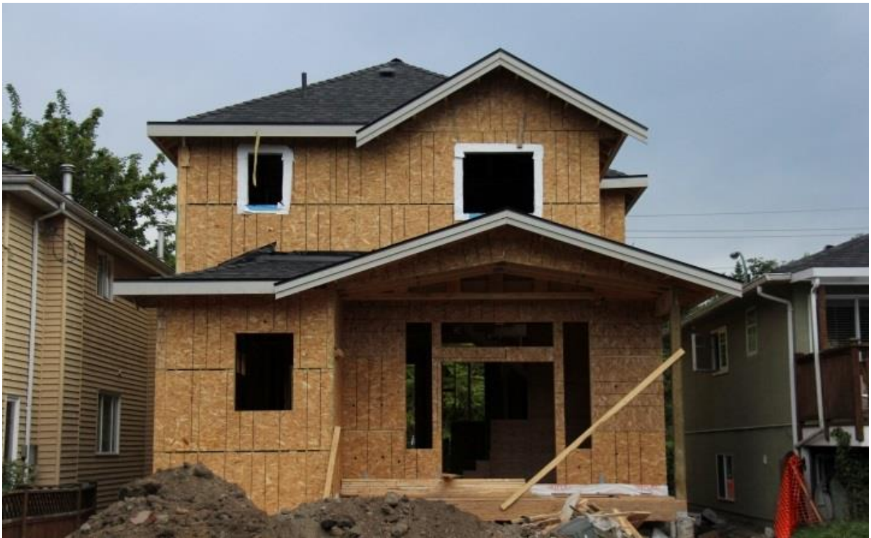
Figure 2.1. A typical two-story single family home under construction in West Point Grey, Vancouver, Canada. Note the large amount of OSB for wall sheathing
