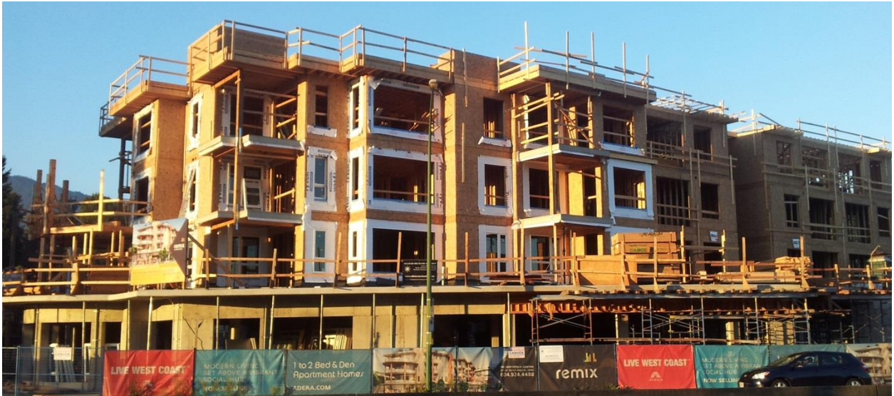
Figure 2.2. A multi-storey building under construction on Marine Drive, North Vancouver, Canada. OSB was used for wall sheathing. The ground floor is typically used for commercial real estate and the upper levels are for medium density residential accommodation
