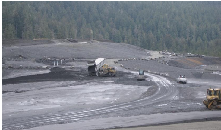
Figure 1. Placing filter pressed tailings at the Greens Creek facility. This stack has been in successful operation since the late 1980s.
