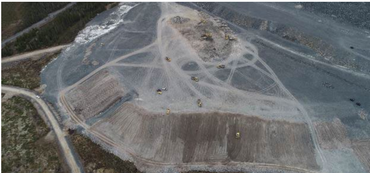
Figure 2. Cover placement during construction of the Test Cover Trial; view looking approximately south.
