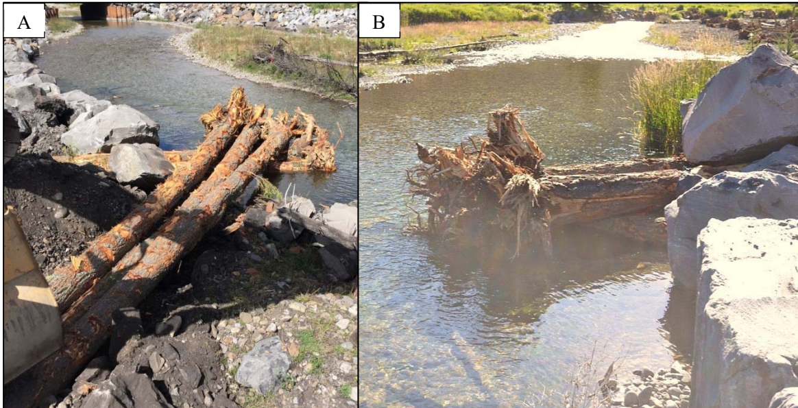
Figure 4 Fording River Rehabilitation near the Concrete Arch Crossing habitat rehabilitation measure example of an instream large woody debris structure (A) during construction (view looking upstream) and (B) after construction (view looking downstream) in September 2016.
