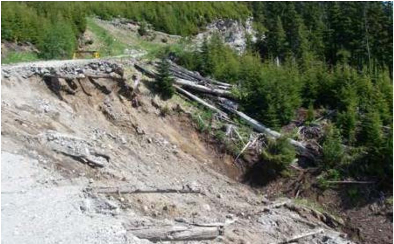
Photograph 2: A large active landslide is the result of poor water management at the road.
