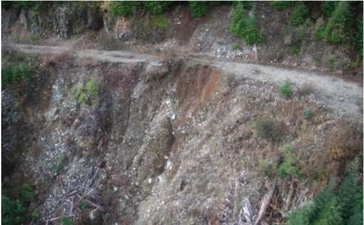
Photograph 3: An abandoned road that has chronic instability as a result of filling across a steep slope including poor water management at the road.
