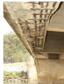
Figure 3: Reinforcement corrosion on bridge deck main girder 1.
