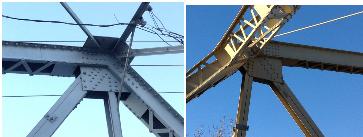
Figure 2: Typical connection details in two steel bridges. a. Non-staggered rivets in the gusset plate; b. Staggered rivets in the gusset plate
