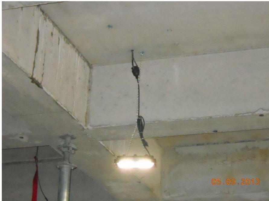
Figure 1: Temporary LED lighting fixture dropped and exposed below ceiling deck (courtesy of Nelson Electric)
