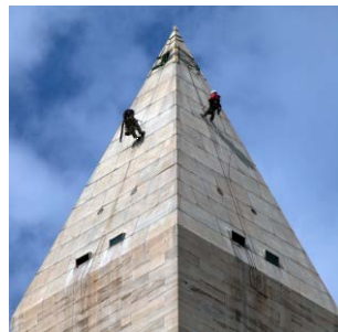
Figure 1: Post-earthquake assessment of Washington Monument (Source: NPS.gov)
